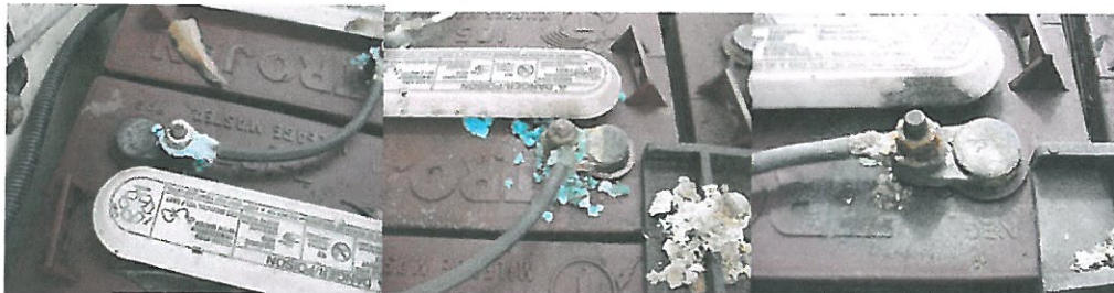
Examples of Poor Maintenance
